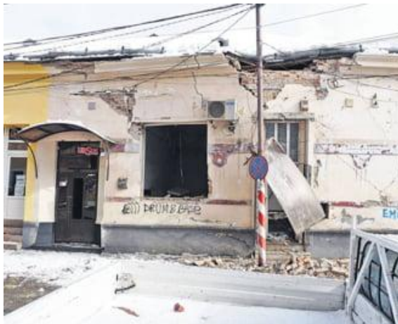
The building in Sighet where the explosion took place [1]
