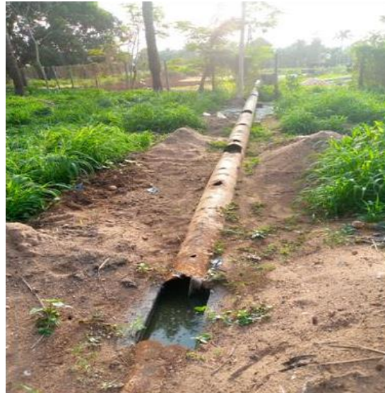
Fig 3: Pitting corrosion in sewer
