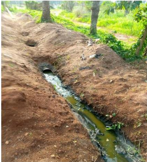
Fig2: Sewer with section of surface lost due to mechanical failure
