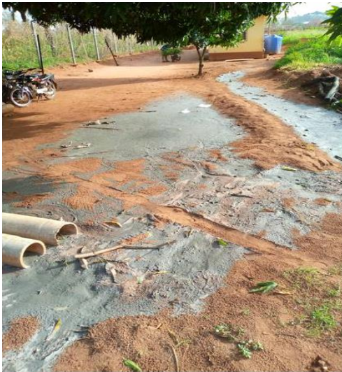
Fig 4: Outflow of sewage in the sewage yard
